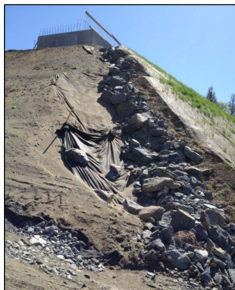
Figure 16. Development on steep slopes and poor erosion control methods can cause erosion and increase the quantity of stormwater runoff. Steep slope development regulations can help prevent some of these impacts. Credit: Vermont Stormwater Program.
