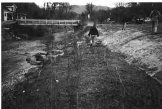
Figure 1. Many streams in the North Carolina mountains and piedmont are incised. The potential for erosion increases as streambank height increases. These incised and eroding streambanks should be graded to include a bankfull bench.
