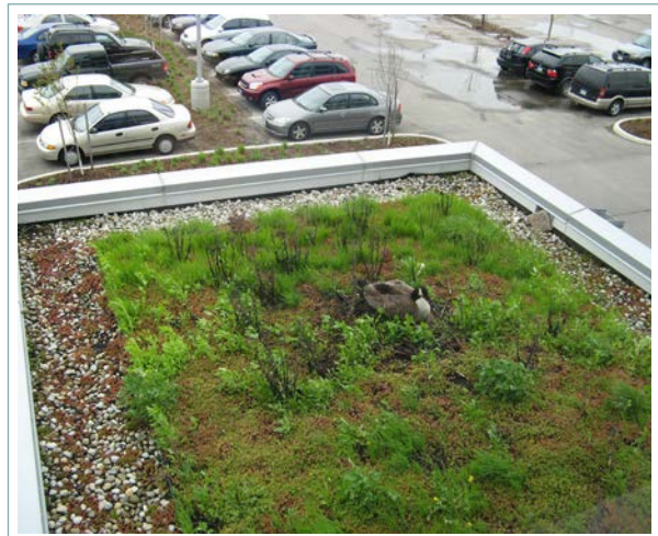
Green roofs can help moderate the urban heat island effect. Photo: S. Woodside/Flickr
