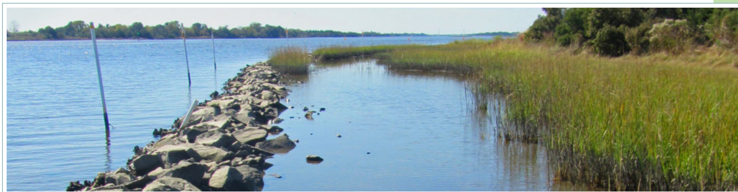
Living shorelines with rock sills can enhance salt marsh resilience to erosion and storms. Photo: Carter Smith
